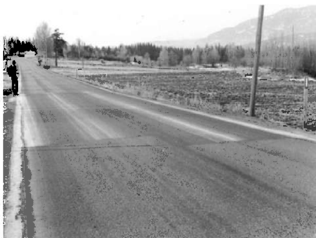
Figure 2. Hoarfrost forming on an insulated road section (Photo: Geir Refsdal)
