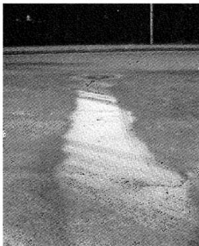
Figure 1. Hoarfrost forming following the excavation for a new pipeline. (Photo: Geir Refsdal)
