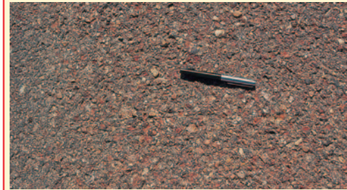
Close-up of the previous photo showing a Single Otta Seal. Note that some of the weak aggregate has been crushed down by traffic, but during the early stage after construction the binder has absorbed the crushed aggregate and a dense water-proof surfacing has been formed. (Botswana).
