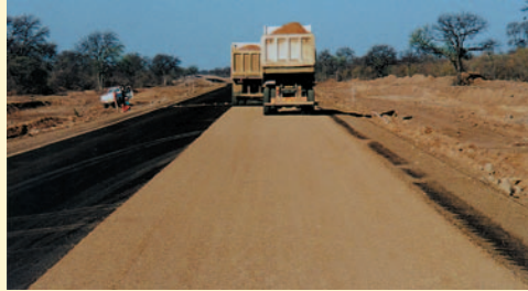
In the absence or in addition to pneumatic rollers, compaction can be successfully carried out by the use of loaded trucks following a pre-determined rolling pattern covering the entire surfaced area. (Botswana).
