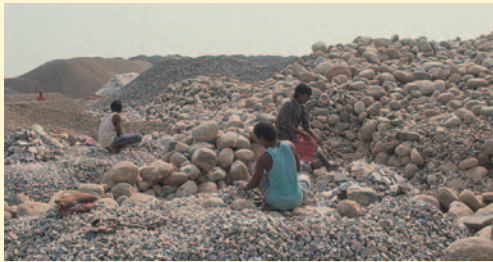
Labour based methods can effectively be used in producing aggregate for use in Otta Seals. (Bangladesh).
