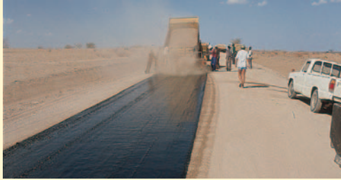
The possible use of natural occurring gravel, including the fines, are some of the factors that favour the use of Otta Seals. (Kenya).
