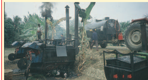
At the Environmental trial Road at Faridpur, the bitumen was both cutback and fluxed in order to give the correct binder consistence. This was successfully carried out by simple but appropriate methods. (Bangladesh).
