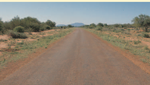
Overview of the same road (Single Otta Seal) after being in service for more than 8 years. (Botswana).
