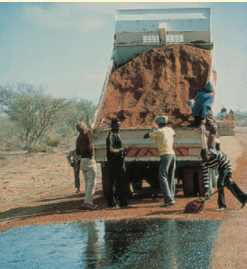
Under the Rural Roads Programme Otta Seals were extensively used, and in combination with labour based work. Natural decomposed granite used as aggregate for Otta Seal was hand screened and applied by hand. (Botswana).
