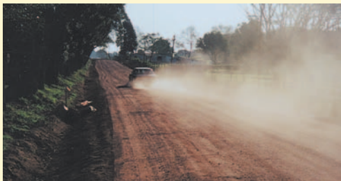
A newly laid Otta Seal (with a high fines content) will for the first 2 - 4 weeks give dust pollution. (South Africa).
