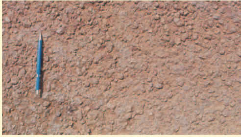
Close-up of an Otta Seal where natural occurring laterite was used as Otta Seal aggregate. (Kenya).
