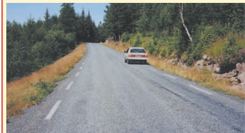
Otta Seal using crushed aggregate on a primary road after 6 years in service. (Norway).
