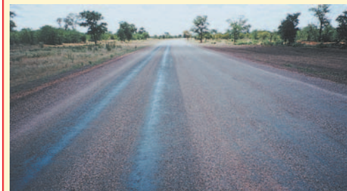
Some bleeding in localised areas and in the wheel paths form a normal part of the curing process. Severe bleeding can be rectified by sand or additional aggregate rolled into the bleeding areas. (Botswana).
