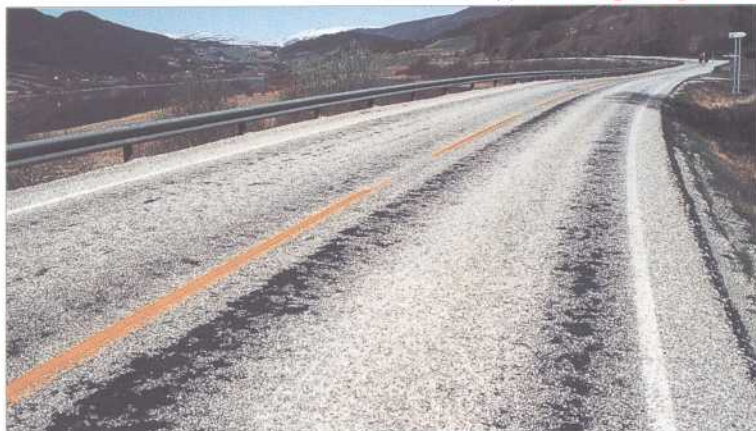
Steinslipp, Alvorlighetsgrad M
