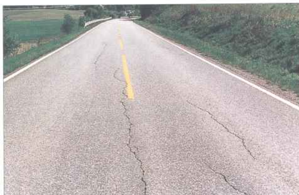
Langsgående telesprekker, alvorlighetsgrad M
